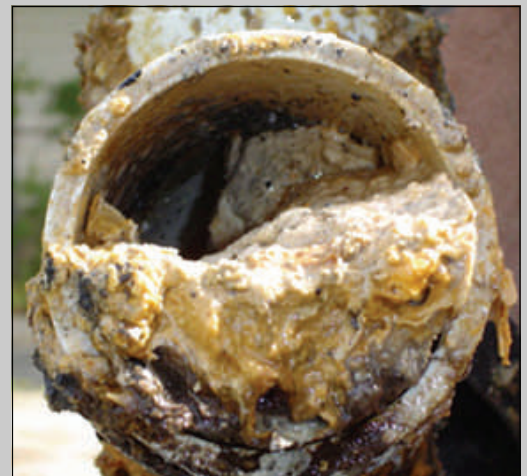
Leaking, Overflowing Grease Traps attract Mice, Insects and Rats
